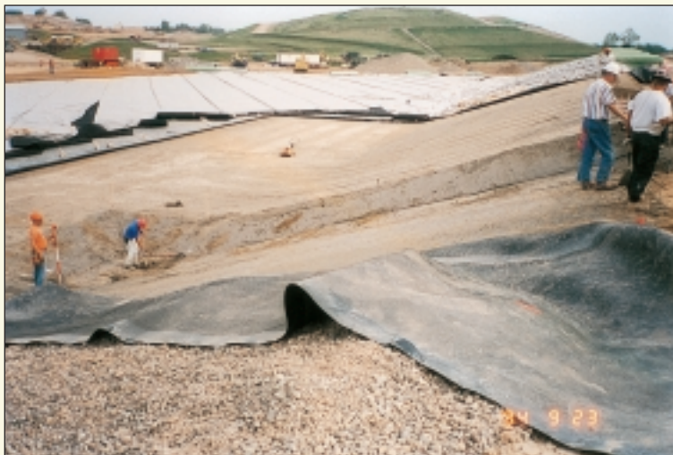
Part of the liner construction of a new landfill at the High Acres Landfill and Recycling Center in Fairport, New York. The hill in the background is a “closed” landfill, which has been through final cover.
