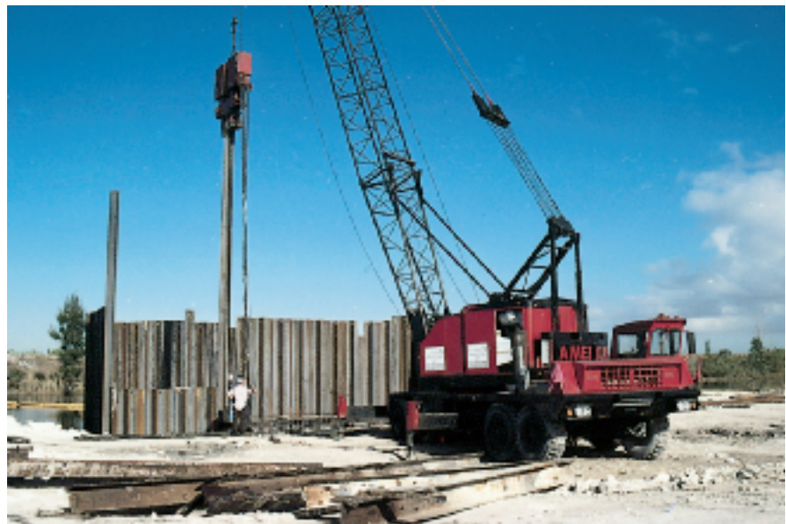
Figure 3-12 In the operation of a pile driver, the gravitational potential energy of the raised hammer becomes kinetic energy as it falls. The kinetic energy in turn becomes work as the pile is pushed into the ground.
