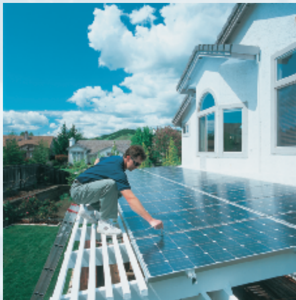
Figure 3-39 Array of solar cells being installed over the back porch of a house in California.
